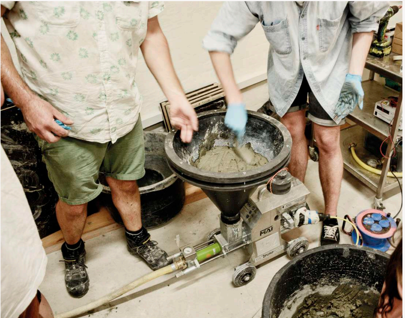
The concrete pump aided by human hands feeding a constant supply of semi-fluid concrete into its rotating auger
