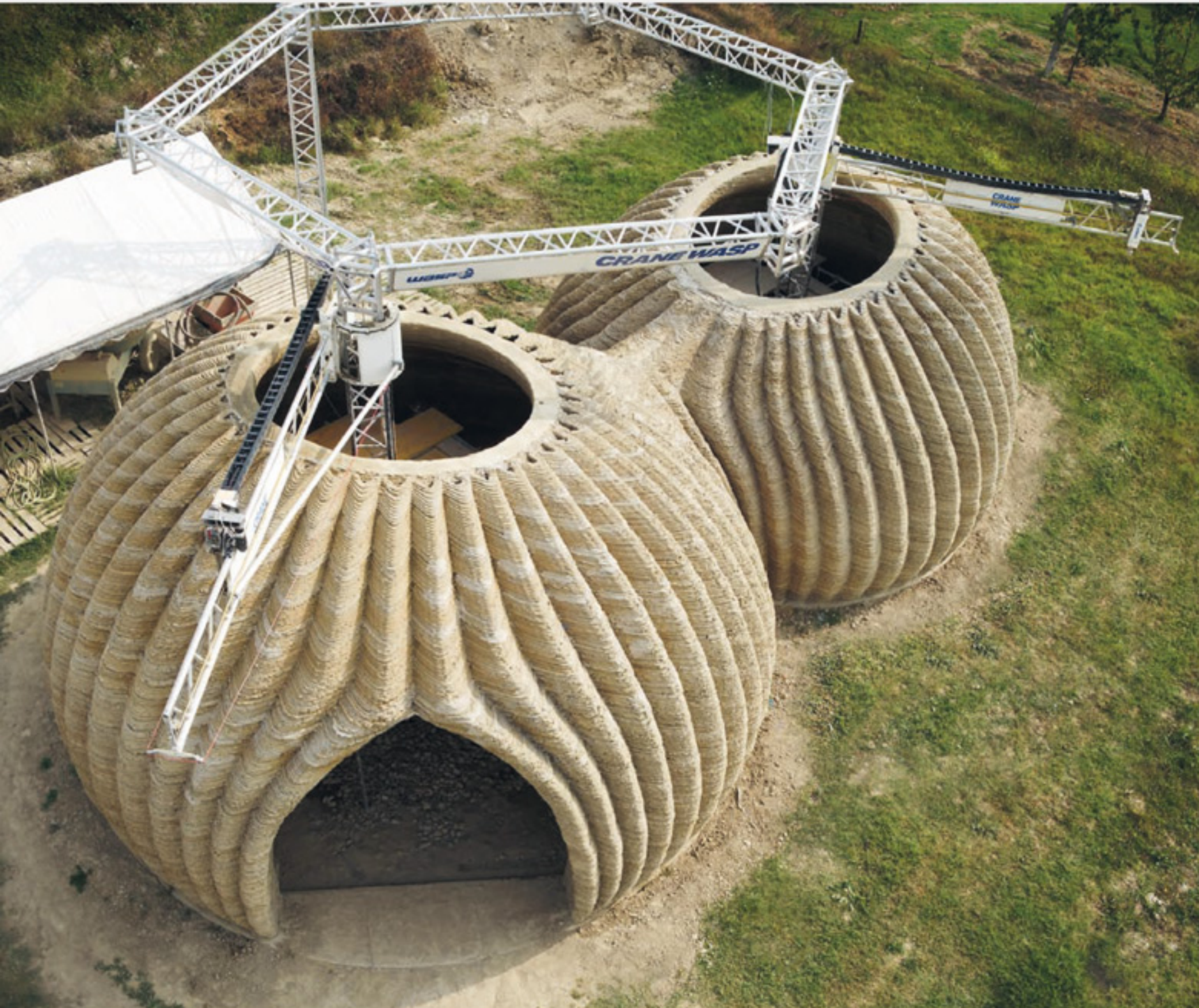
Figure 5: A network of modular WASP printers allowed for multiple areas of the structure to be printed simultaneously without collision
