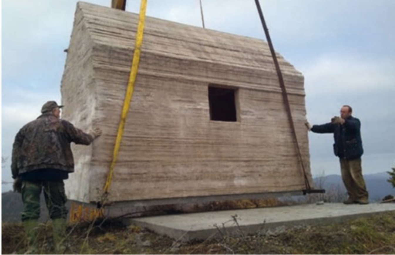
Figure 11. Una Casa Tutta D'un Pezzo: The use of a Binder Jetting process in construction was illustrated by Enrico Dini Image Source: Reproduced with the permission of Enrico Dini
